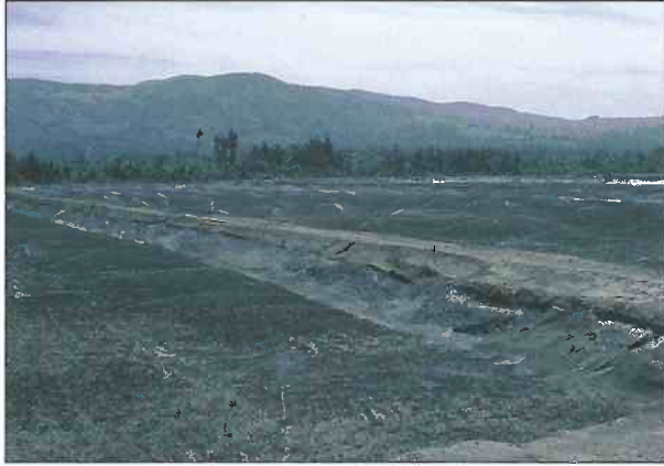
Figure 6.—A newly constructed bed ready for planting, showing perimeter ditches and dike.
